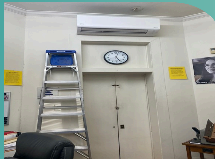
Sa Alliance for Teachers mini split installation
